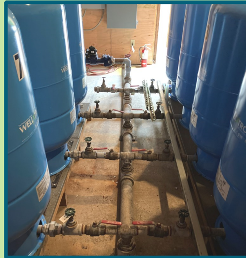
Sierra Treatment System
