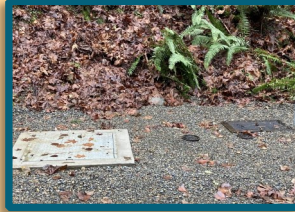
PRV above ground view
