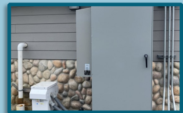
Well Motor Control Panel
