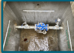
View looking down into PRV vault
