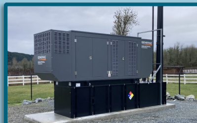
Well Site Generator
