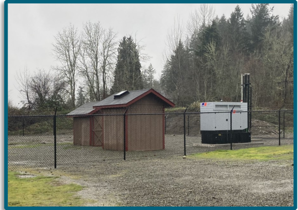
New generator for Sierra 2022
